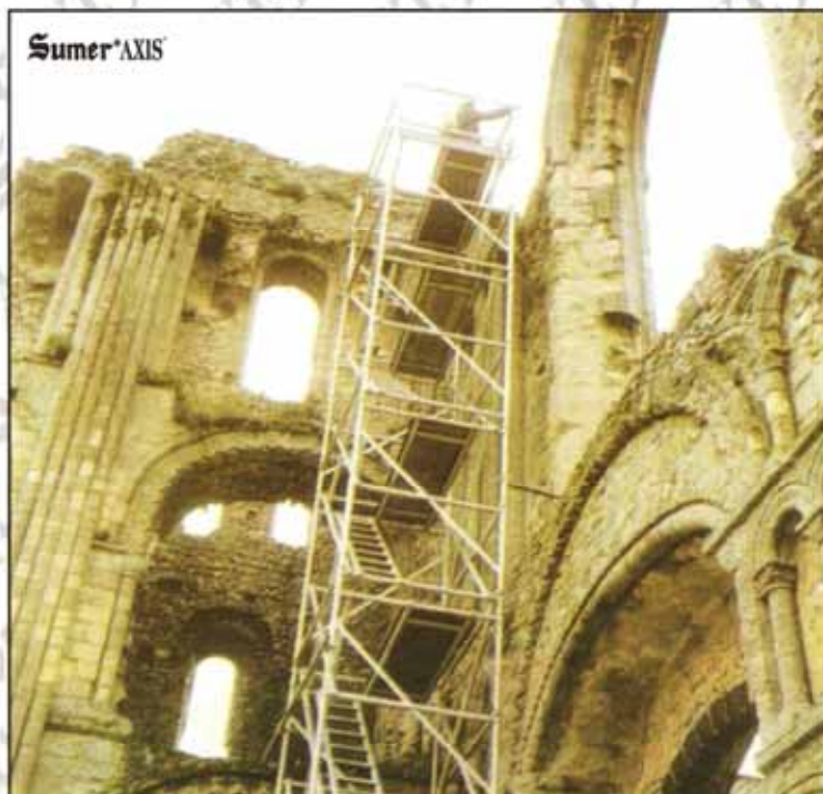
Maintenance - Mobile Access Platform
